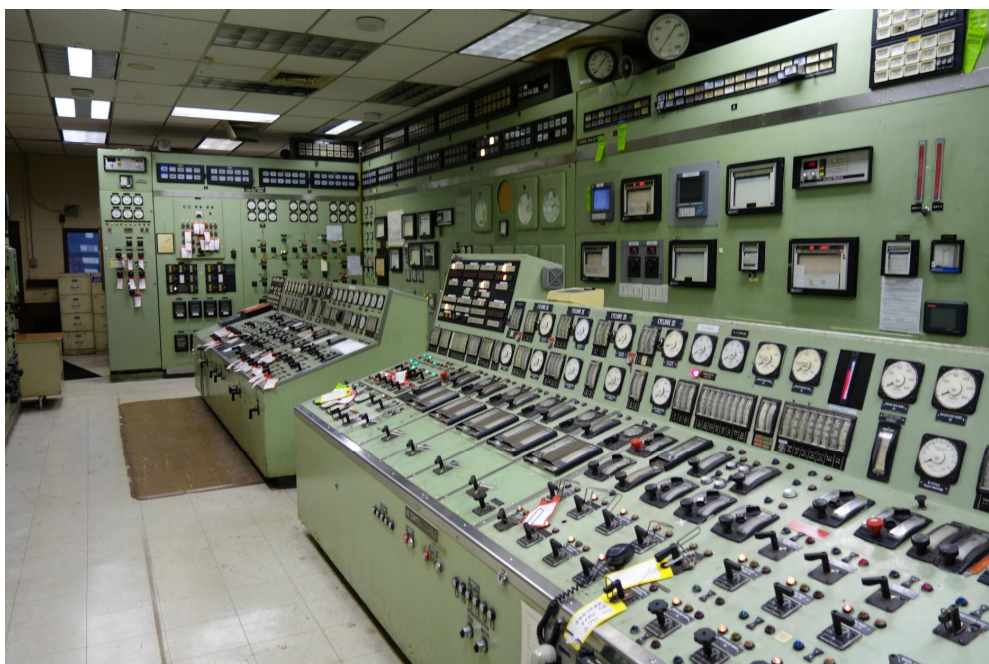
Coal Power Plant Ref: http://power-controlsystem.com/
